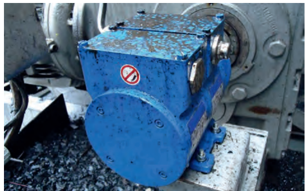
Nachher: U-ONE-SAFETY-Compact direkt angebaut / After: U-ONE-SAFETY-Compact directly mounted
